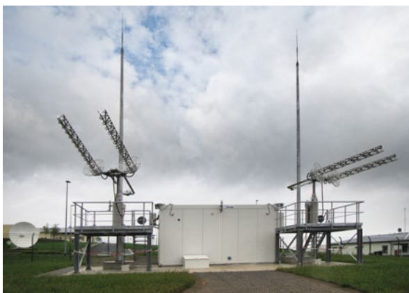
The UHF DAMA control station in Gerolstein was handed over by OHB representatives to the BAAINBw and the user Bundeswehr during a celebration Source: OHB System AG
